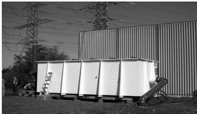
Fig. 2 A 950-cfm-capacity modular biofilter system treats air emissions from a wastewater pumping station. The biofilter system is filled with a manufactured synthetic medium
